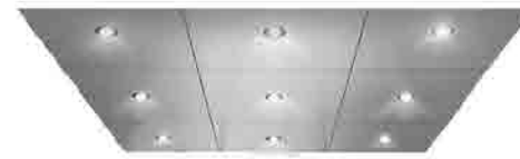
LED downlights recessed in canopy
